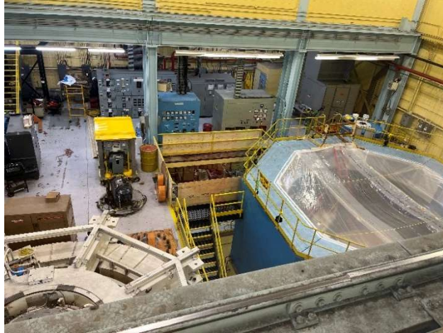
Figure 1: Hinds Lake Generating Unit 47
